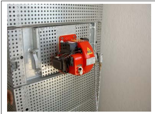
Picture 34: Burner stand in incineration position
