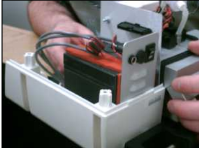
Properly Installed panel
