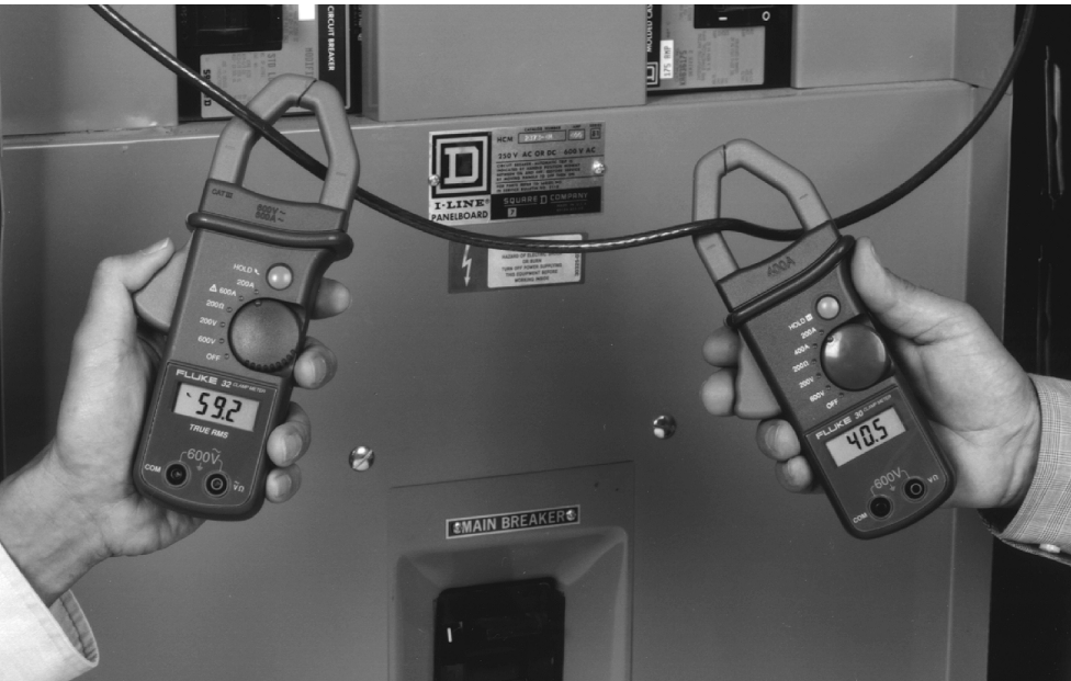
Figure 1. One current—two readings. Which do you trust? The branch circuit above feeds a non-linear load with distorted current. The True-rms clamp reads correctly but the average responding clamp reads low by 32%.
